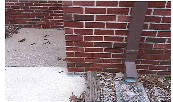
Masonry tuckpointing needed near downspout
