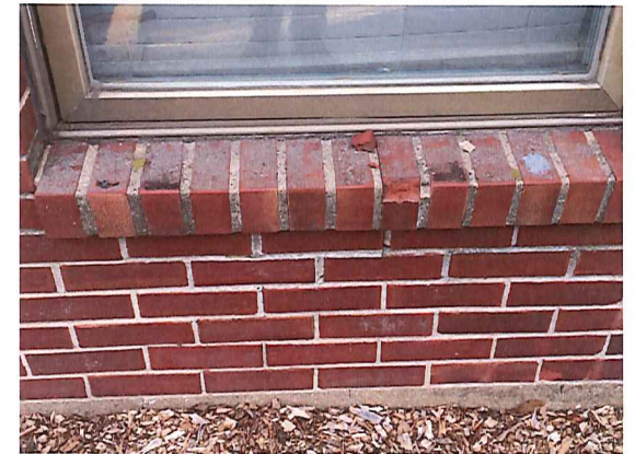
Deteriorated brick rowlock
