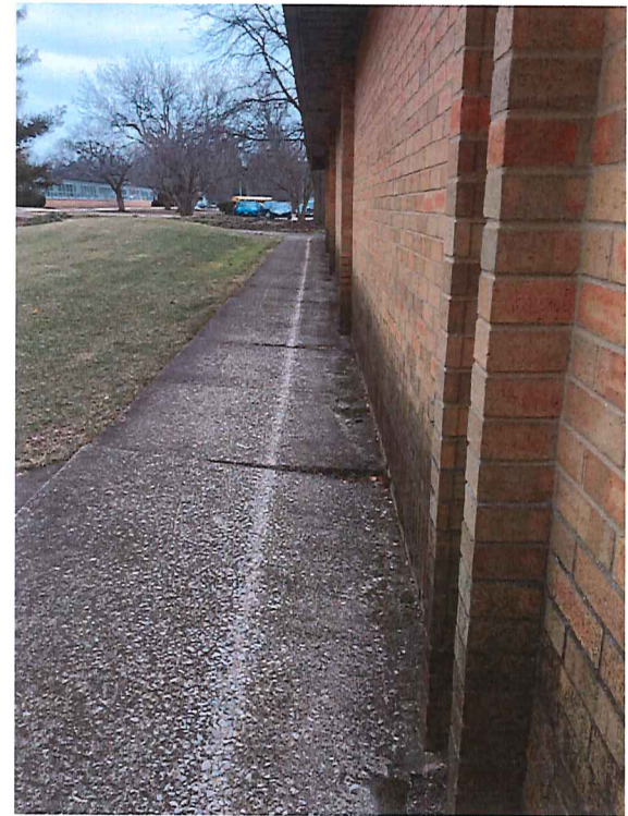
Pavement settlement at north wall
