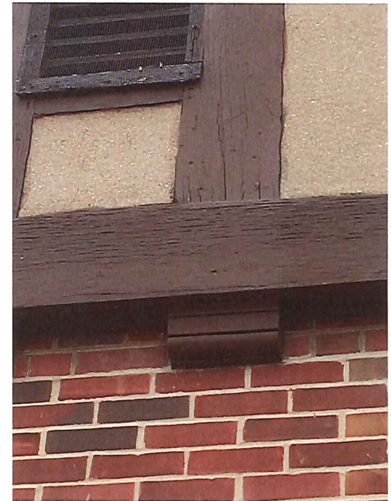
Deteriorated wood trim
