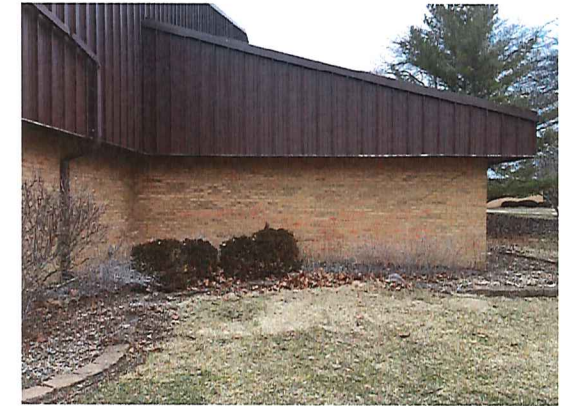
Stair-stepped masonry crack
