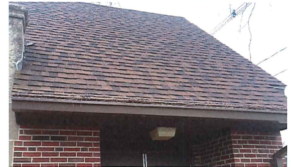
Gutters need cleaning
