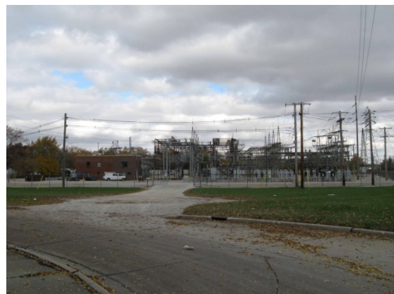
Figure 3.3: The northeastern corner of the Bristol Place neighborhood is bordered by an energy substation.
