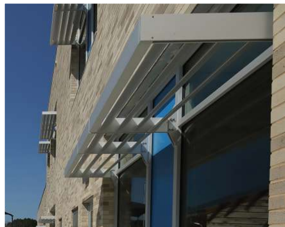
Horizontal Sun Shading System
