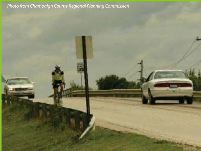
The existing Windsor Road bridge over Interstate 57 does not accommodate bicycles or pedestrians creating a hazardous situation for crossing. Bridge replacement should adhere to adopted City and State policies for "complete streets."
